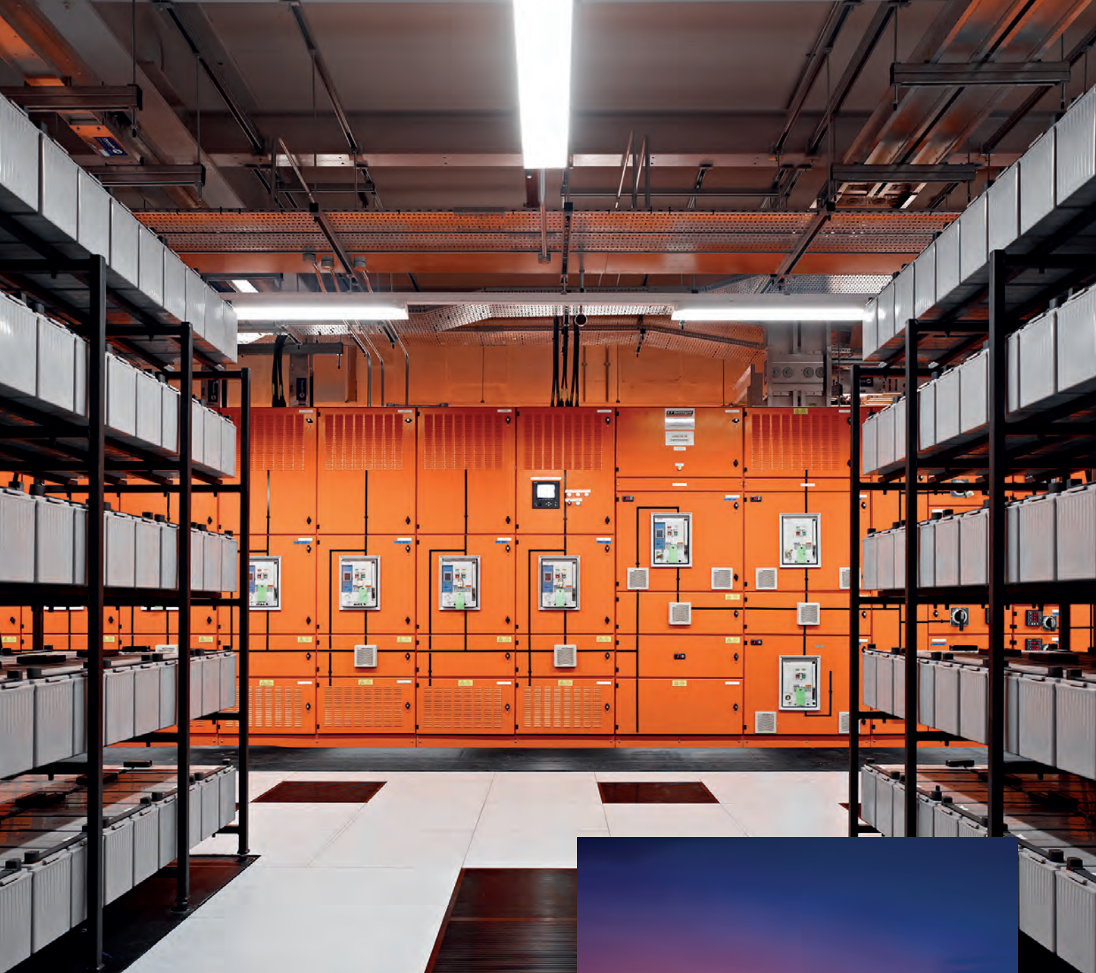
[Telehouse Data Centre, London. 199 TemPower 2 ACBs, 423 TemBreak 2 MCCBs.]
