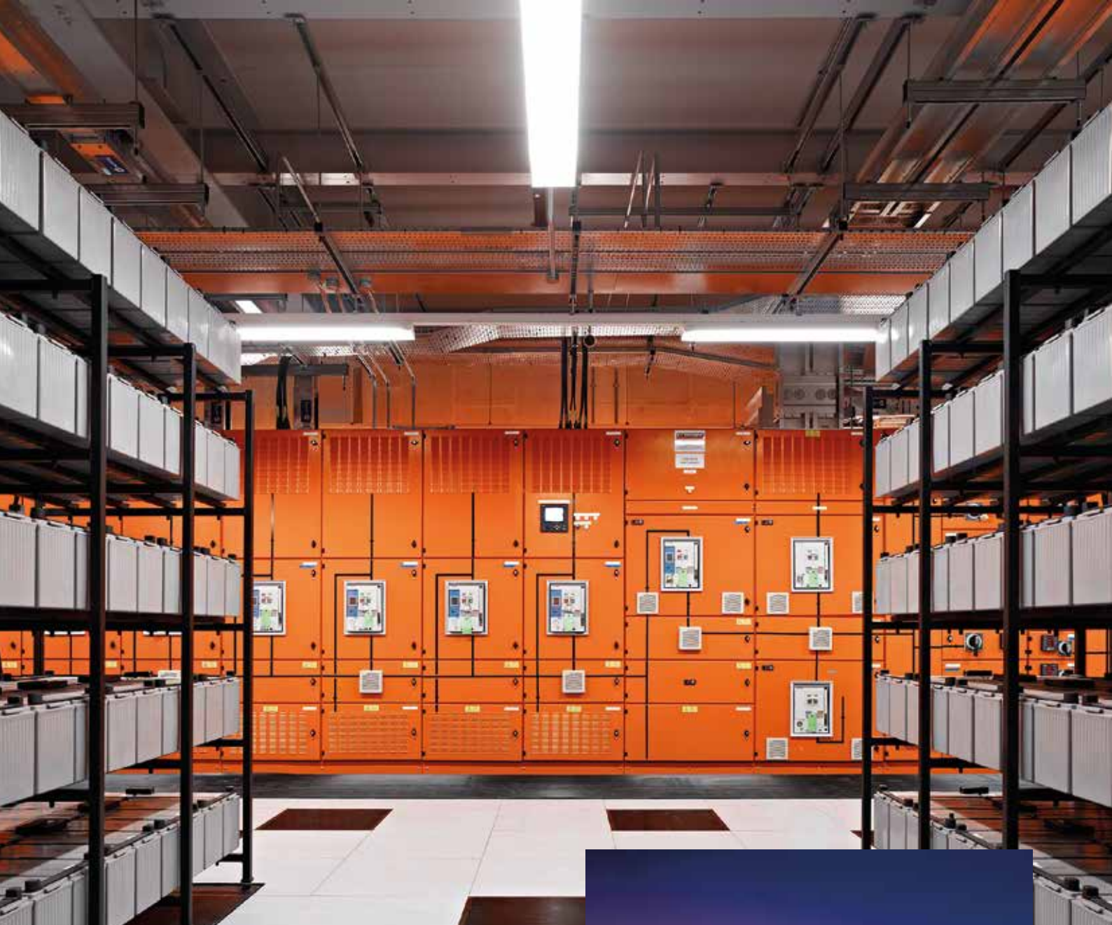
[Telehouse Data Centre, London. 199 TemPower 2 ACBs, 423 TemBreak 2 MCCBs.]
